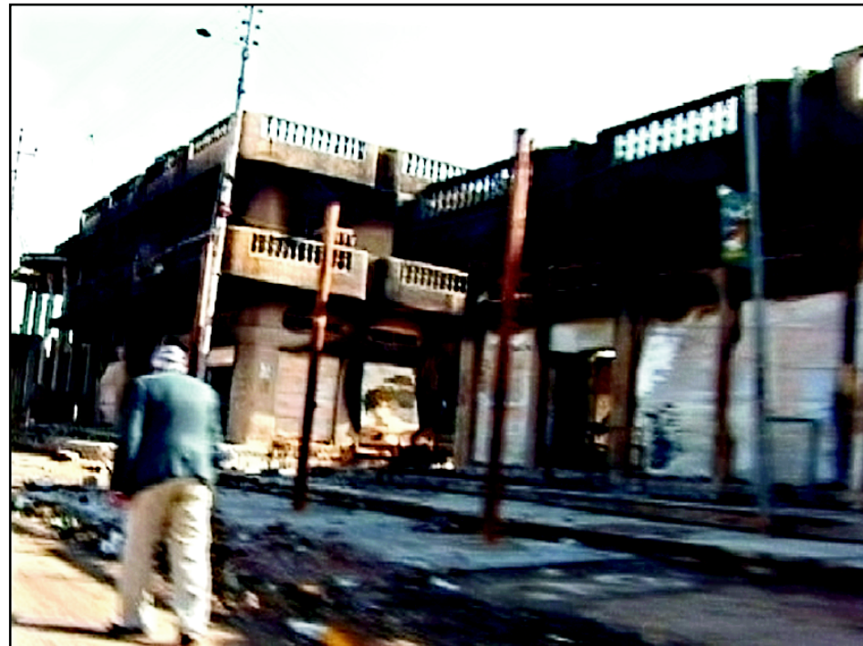
AN OLD MAN walks home passed a blown out building in Falluja Iraq after the second siege there led by American forces.
